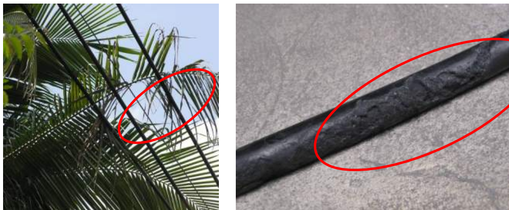
Figure 5: Insulated cable intermittently touching a tree (left) leads to deterioration of insulation (right).
