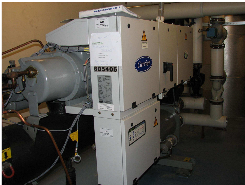
Figure 2 Example of a heat pump at Zuidpoort (the Netherlands) [4]
