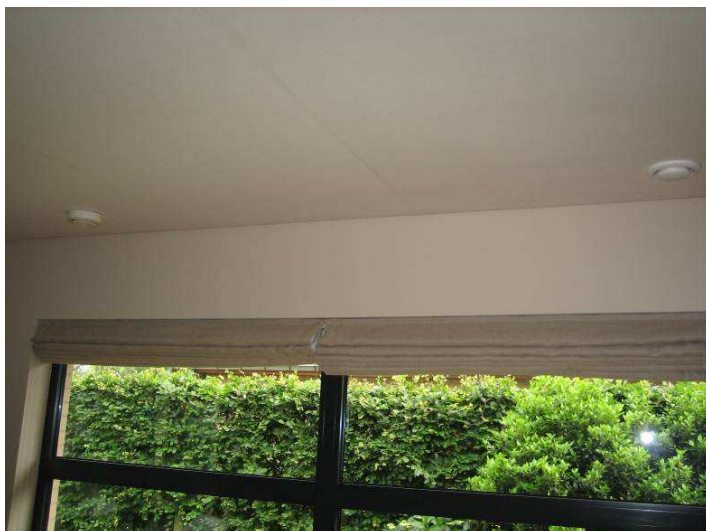
Figure 4 - The ventilation system
