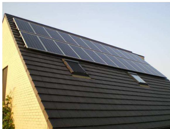
Figure 5 - The PV panels on the roof
